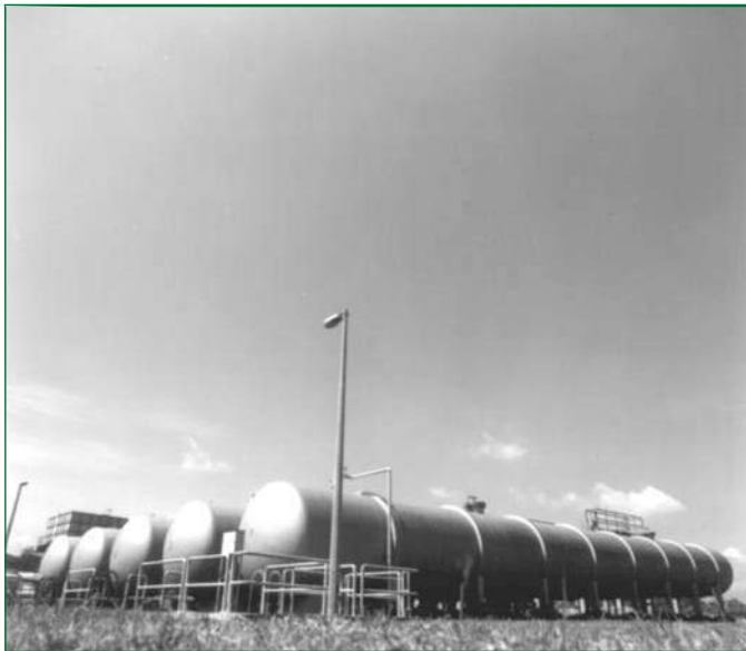
Surge Vessel at Sungai Selangor Water Treatment Plant
